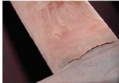
4. Repeated quench of hot tube caused by leaking attemperator control valve resulted in cracking from thermal-mechanical fatigue
