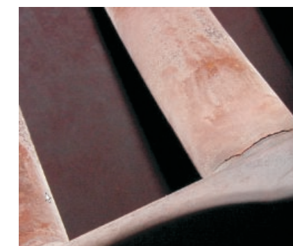
1. Cracking occurred at this tube-to-header connection in an HRSG reheater operating behind an F-class gas turbine. Both the tubing and piping are Grade 91 material, which many assumed would be a panacea for HRSG troubles
