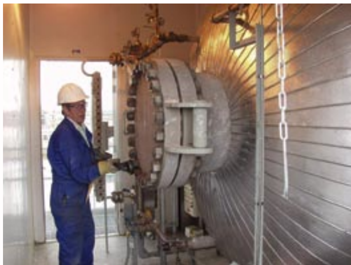
4. Proper shutdown and layup of the HRSG is needed not only to minimize corrosion during the shutdowns, but to reduce delays during the subsequent startups and ensure top performance during the operating periods
