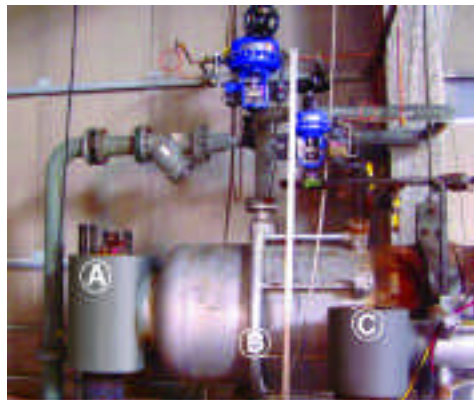
1. Steam-turbine bypass system is being installed at a 250-MW, 1-by-1 combined-cycle plant. HP (A) and IP (C) valve bodies await receipt of actuators and valve gear. B is spray water manifold for HP desuperheater. Desuperheated steam is routed to sparger in steam-turbine exhaust duct
